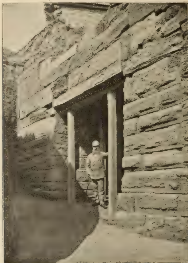
FIG. 334. Gates ( E on Plan VII. v. inset) in the Greek Wall of Chersonese. Eight courses of 1st period, one of 2nd; above, Roman with threshold of postern. The gate was 3·87 m. broad, the passage way 8·39 m. long. Just within the entrance are portcullis-grooves and 5·33 m. from the face of the wall are projections reducing the opening to 2·12 m. To the east of the gate inside was a stair to go up on the wall. Three water runnels meeting give the directions of streets, two "back of the walls," one towards the Acropolis and one towards the harbour (Fig. 338). At a lower level than all this was a sepulchral monument 2·40 m. square as it were a pyramid with three steps ( CR. 1900, p. 21, f. 43). The jambs of the gate shewed no signs of any traffic having passed through it.
